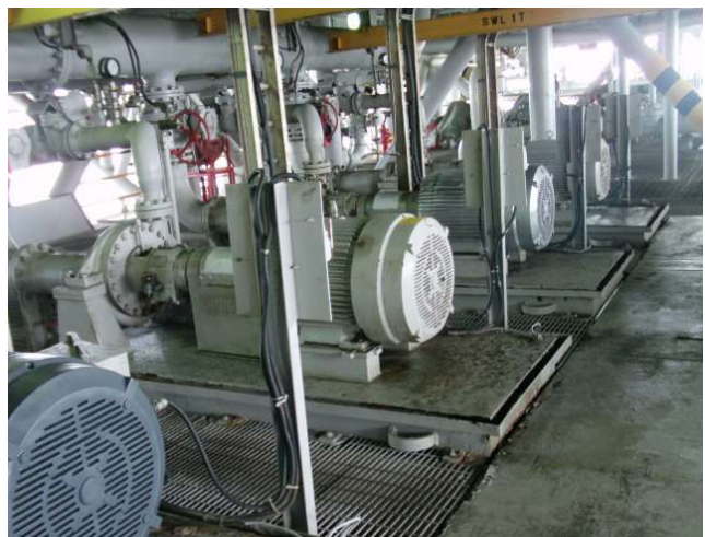
Pump Maintenance Operations
