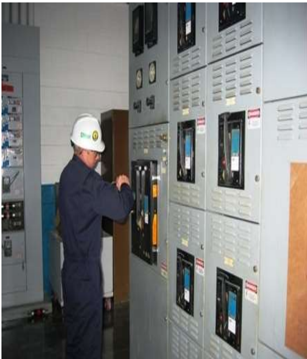
ELECTRICAL EQUIPMENT VERIFICATION PROJECT FOR GPL
